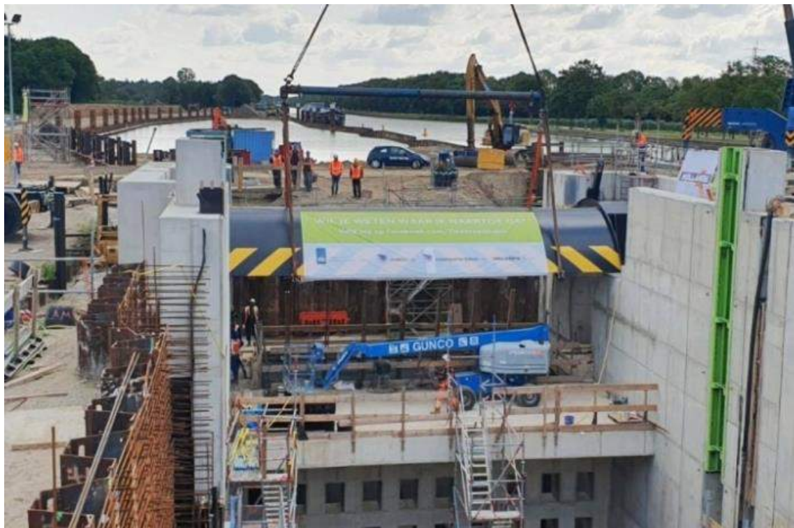
Fig. 1-9-2 Construction design of a stemless gate for a lock gate of the Saitama Lock. The gate is made of a stemless gate (Fig. 1-9-1)
