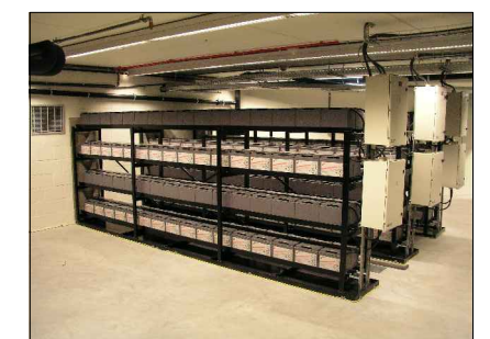
4 Noodstroombatterijen UPS Batteries de secours UPS
