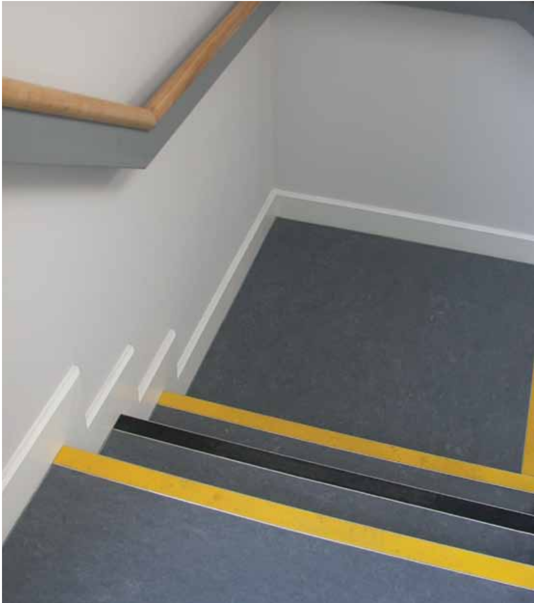
Image 3.1 Example of stairs with non-slip applied nosing.
