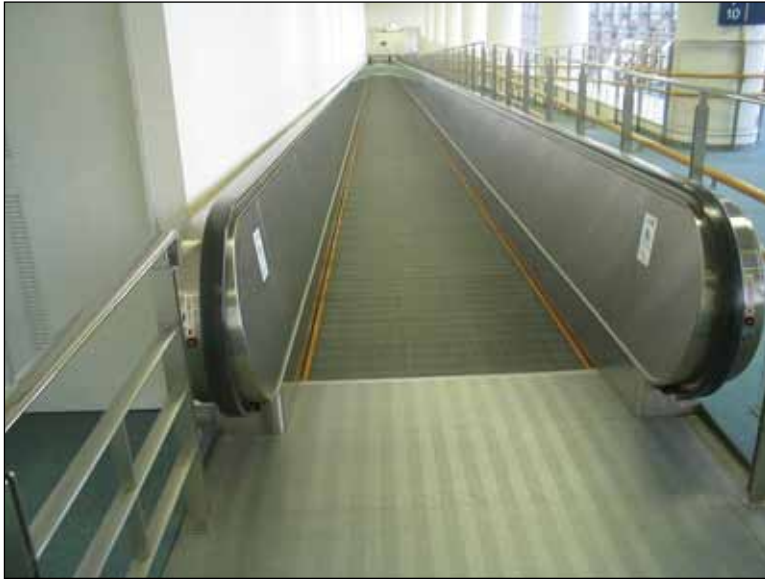
Image 3.24 Example of inclined travelator.
