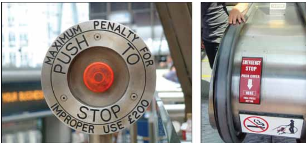
Image 3.21 and 3.22 Examples of escalator emergency stop buttons.
