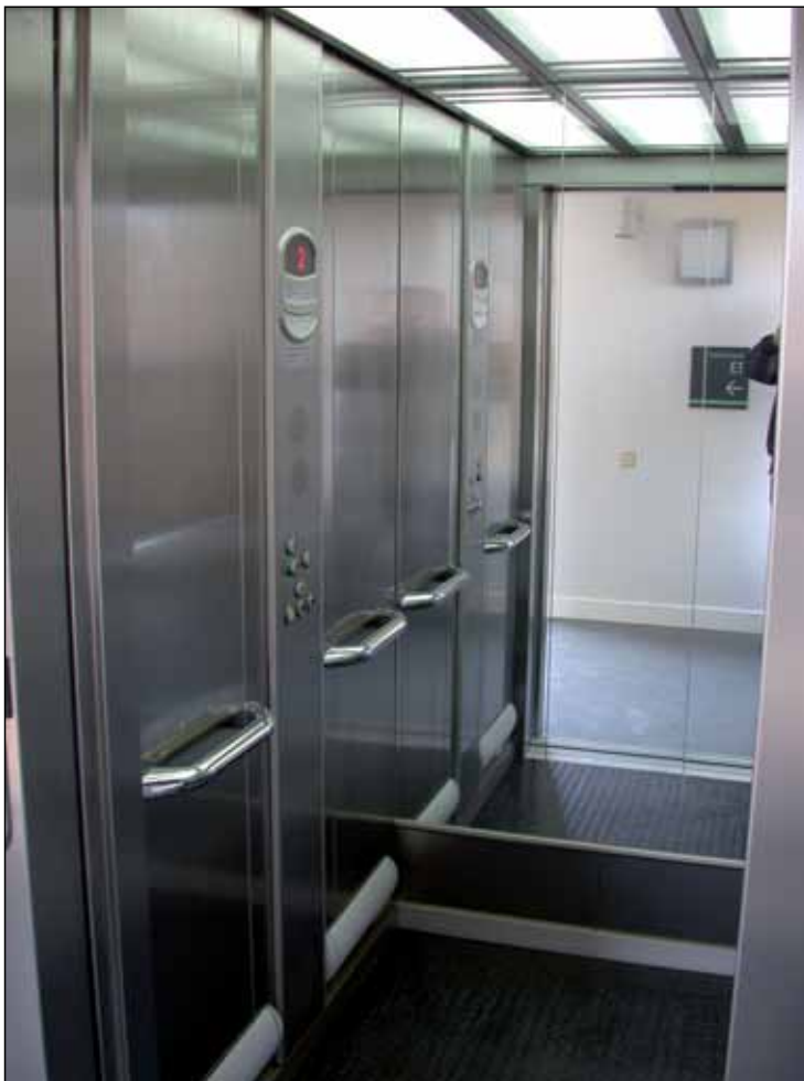
Image 3.10 Example of lighting in a lift.
