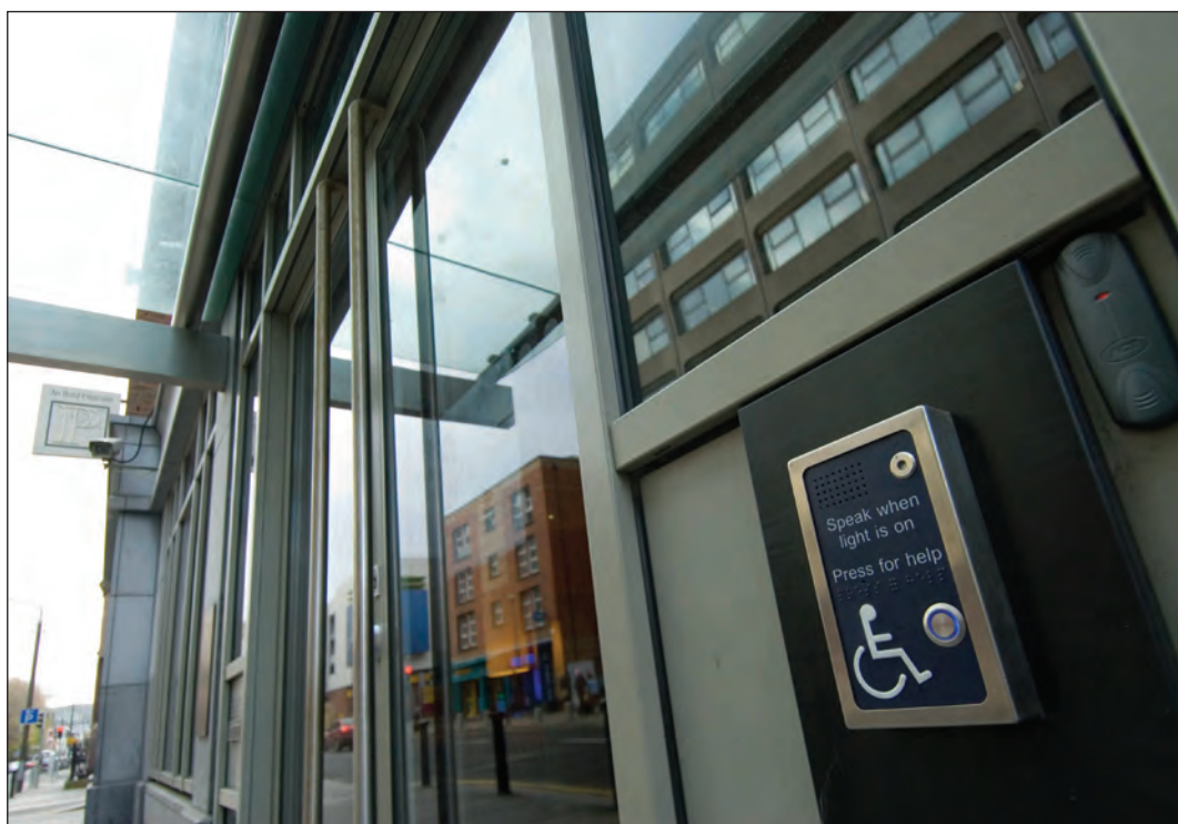
Image 2.31 Example of intercom access system.
