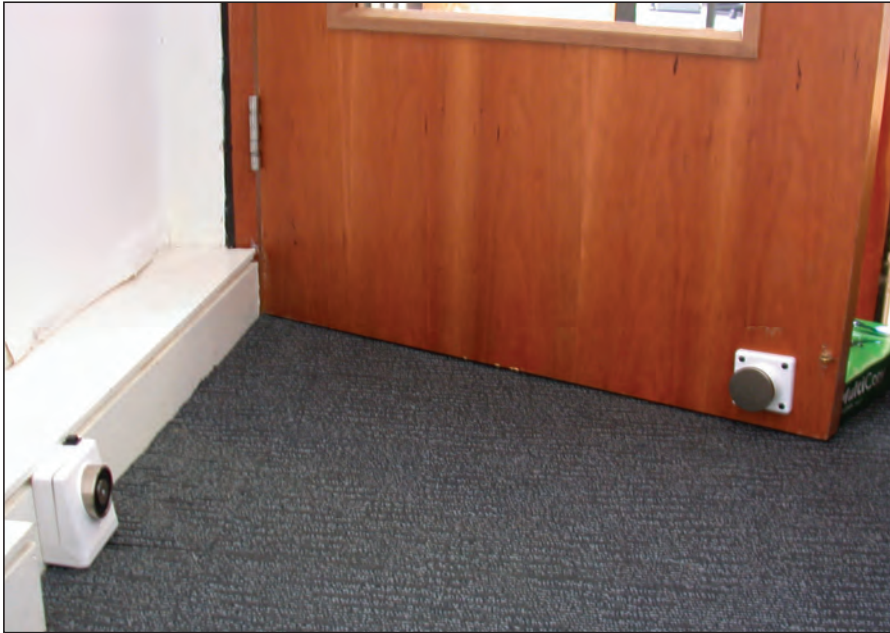
Image 2.25 Example of electromagnetic hold-open device.
