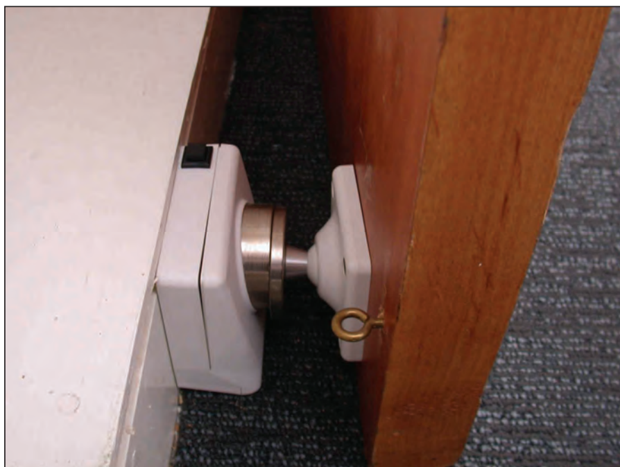
Image 2.24 Example of electromagnetic hold-open device for doors in use.
