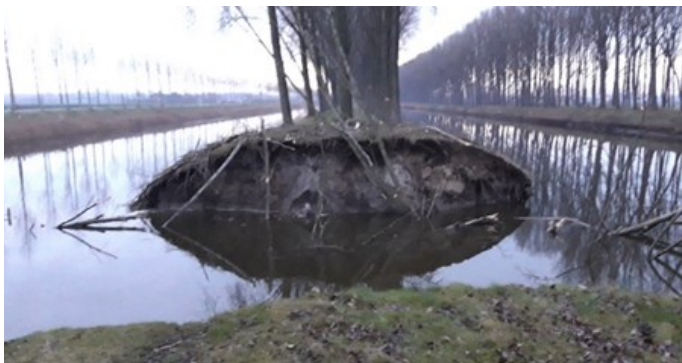
Figure 4: Breached central levee, end 2018.
