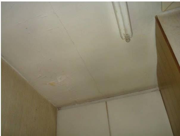
barst in plafond
