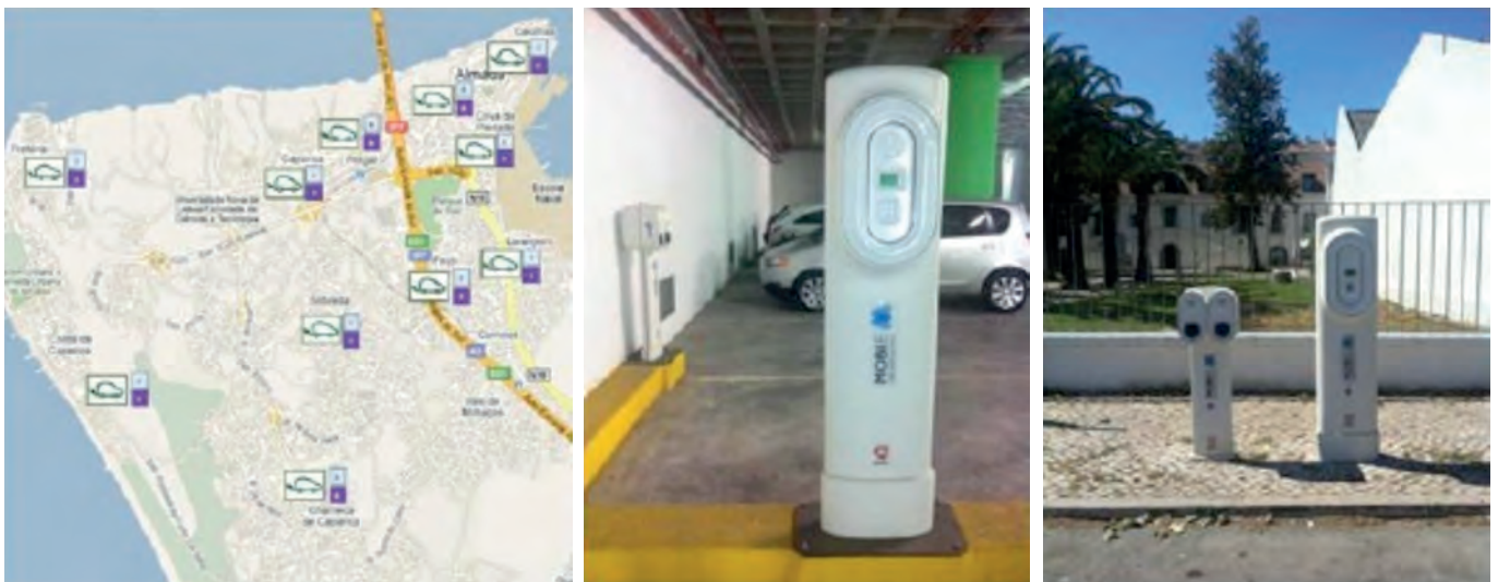
Figure 16 – EV charging points location and devices at Conde Ferreira parking and on the street
